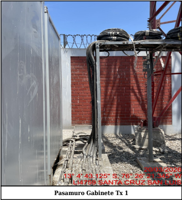
Pasamuro Gabinete Tx 1
