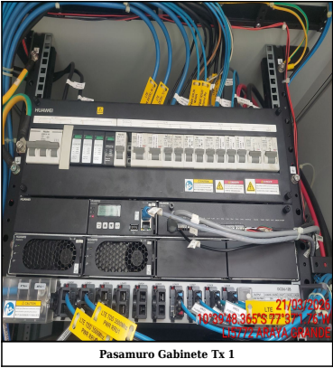
Pasamuro Gabinete Tx 1
