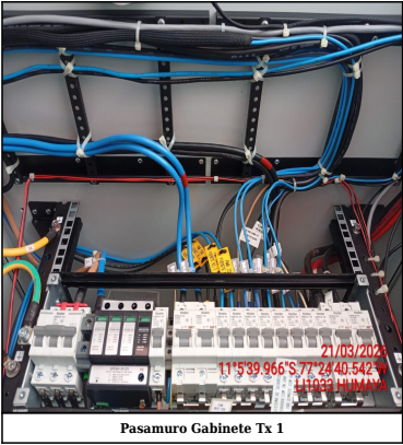
Pasamuro Gabinete Tx 1
