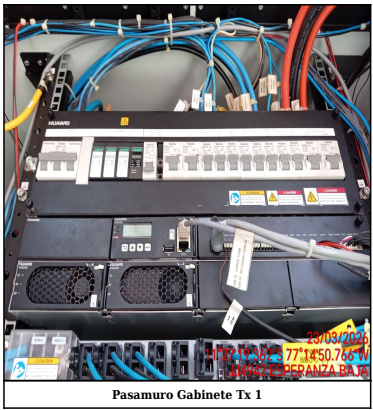
Pasamuro Gabinete Tx 1
