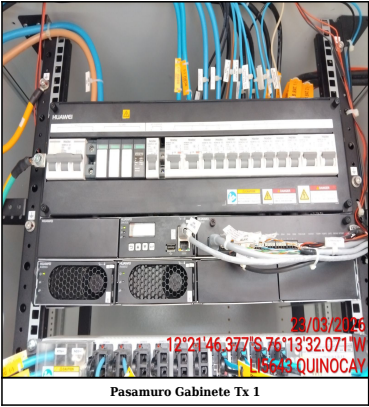
Pasamuro Gabinete Tx 1
