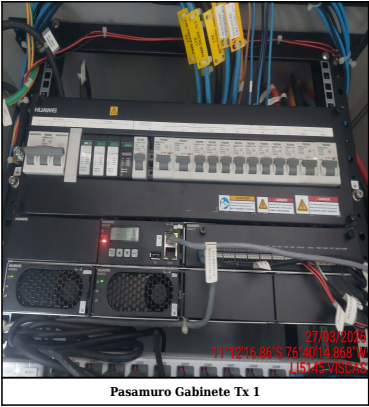
Pasamuro Gabinete Tx 1
