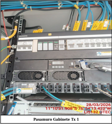
Pasamuro Gabinete Tx1
