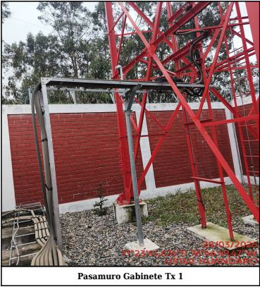
Pasamuro Gabinete Tx 1
