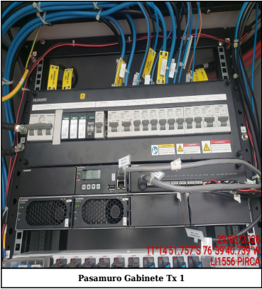
Pasamuro Gabinete Tx 1
