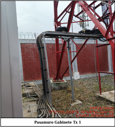
Pasamuro Gabinete Tx 1
