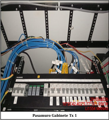
Pasamuro Gabinete Tx 1
