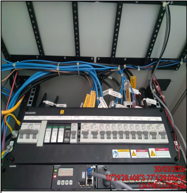
Pasamuro Gabinete Tx 1
