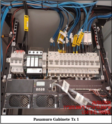
Pasamuro Gabinete Tx 1
