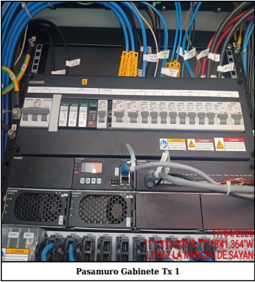
Pasamuro Gabinete Tx 1
