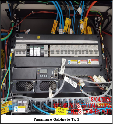
Pasamuro Gabinete Tx 1
