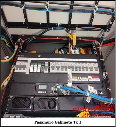
Pasamuro Gabinete Tx 1
