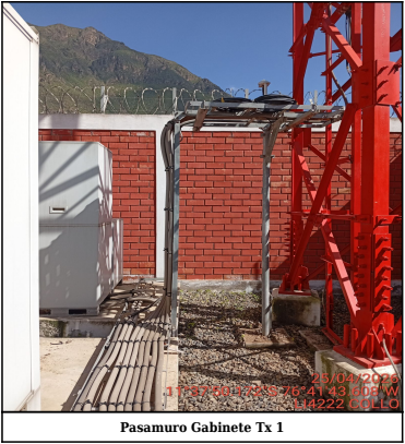
Pasamuro Gabinete Tx 1
