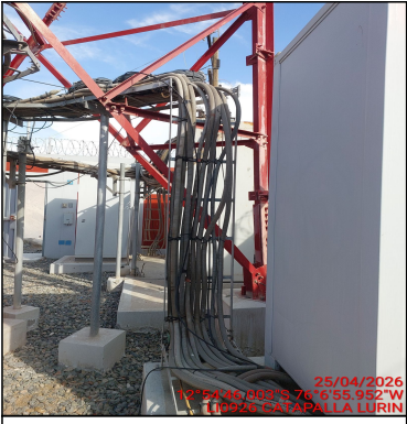
Pasamuro Gabinete Tx 1
