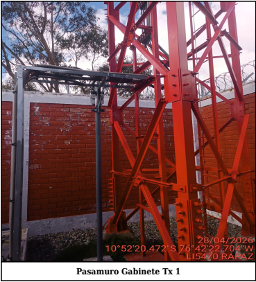
Pasamuro Gabinete Tx 1
