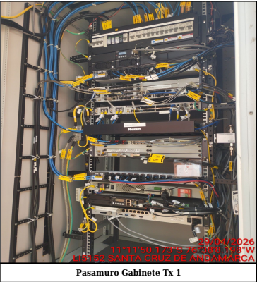
Pasamuro Gabinete Tx 1
