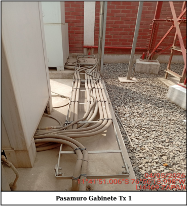
Pasamuro Gabinete Tx 1
