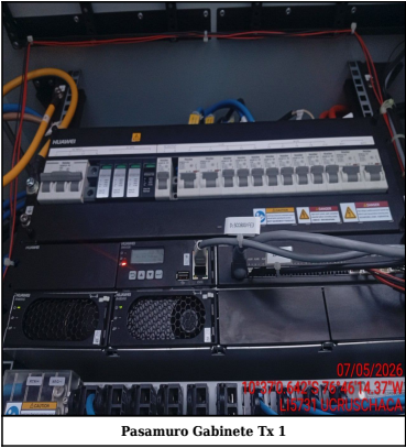
Pasamuro Gabinete Tx 1
