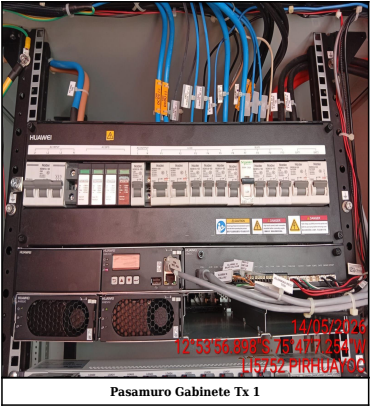
Pasamuro Gabinete Tx 1
