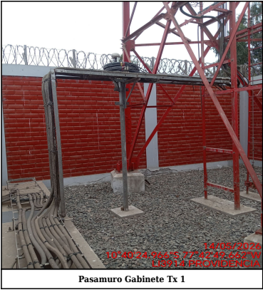
Pasamuro Gabinete Tx 1
