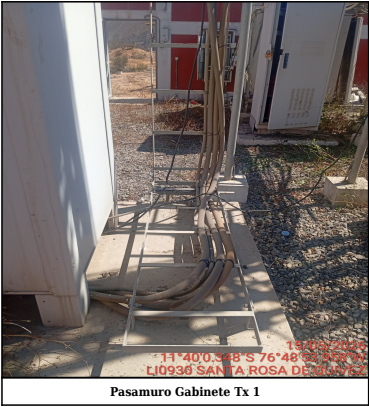
Pasamuro Gabinete Tx 1
