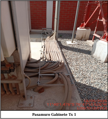
Pasamuro Gabinete Tx 1
