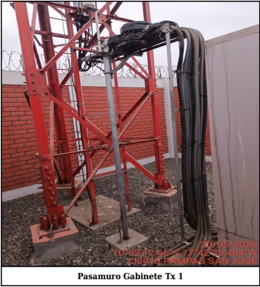
Pasamuro Gabinete Tx 1
