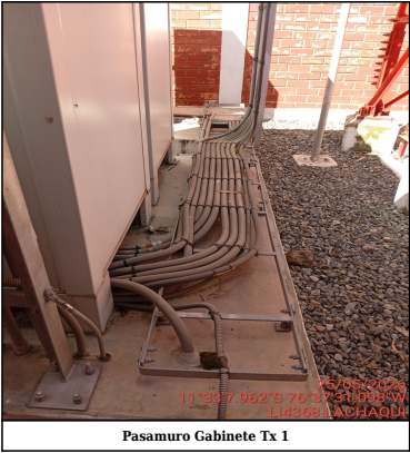
Pasamuro Gabinete Tx 1
