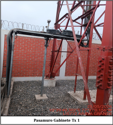
Pasamuro Gabinete Tx 1
