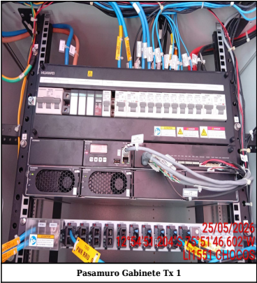
Pasamuro Gabinete Tx 1
