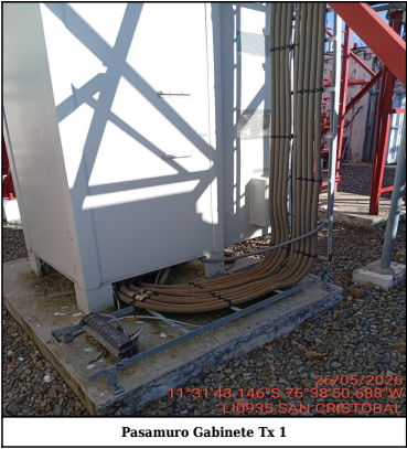
Pasamuro Gabinete Tx 1
