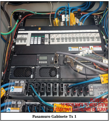
Pasamuro Gabinete Tx 1
