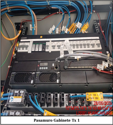
Pasamuro Gabinete Tx 1
