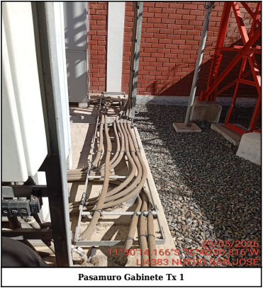
Pasamuro Gabinete Tx 1
