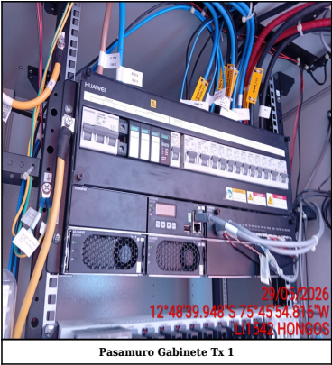
Pasamuro Gabinete Tx 1
