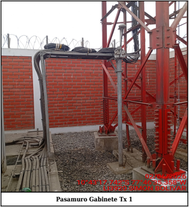
Pasamuro Gabinete Tx 1
