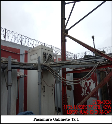
Pasamuro Gabinete Tx 1
