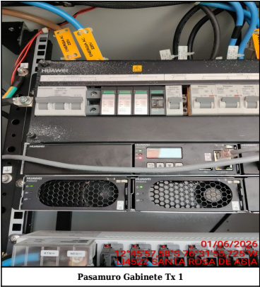
Pasamuro Gabinete Tx 1
