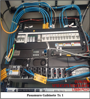
Pasamuro Gabinete Tx 1
