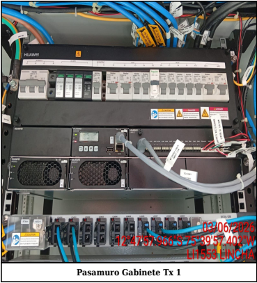
Pasamuro Gabinete Tx 1
