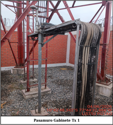
Pasamuro Gabinete Tx 1
