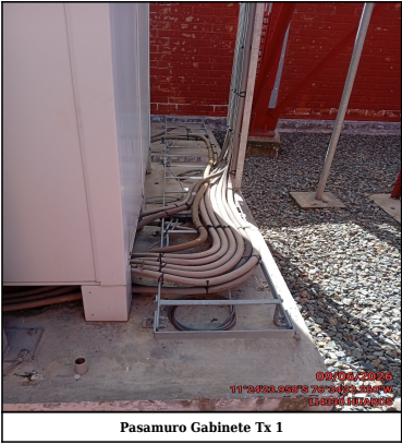
Pasamuro Gabinete Tx 1
