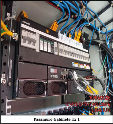
Pasamuro Gabinete Tx 1
