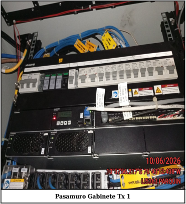
Pasamuro Gabinete Tx 1
