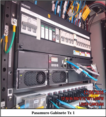
Pasamuro Gabinete Tx 1
