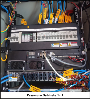
Pasamuro Gabinete Tx1
