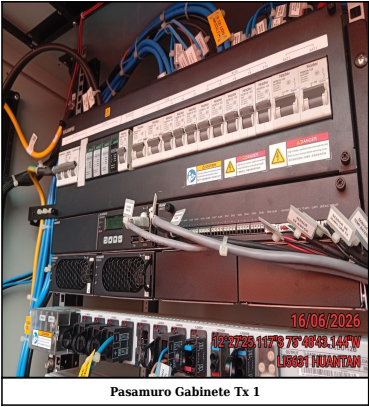
Pasamuro Gabinete Tx 1
