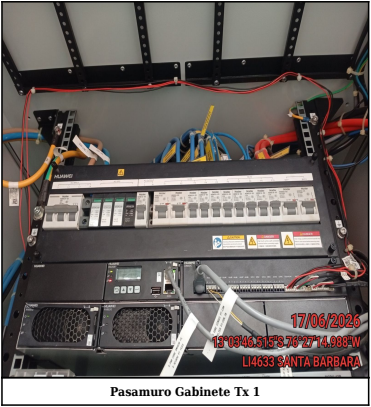
Pasamuro Gabinete Tx 1
