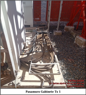
Pasamuro Gabinete Tx 1
