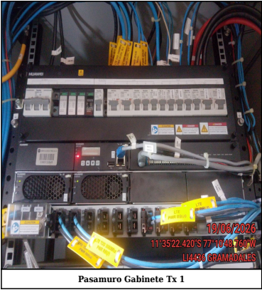
Pasamuro Gabinete Tx 1
